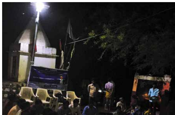
Solar Street Light installed in Salhedanda, Mandla district, Madhya Pradesh
