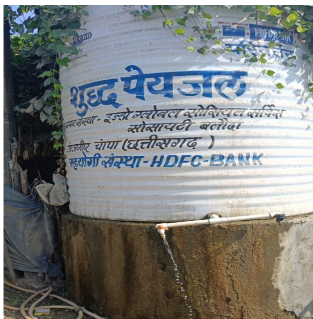
7 Drinking water tank - Puren village
