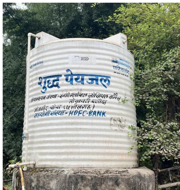
8 Drinking water tank - Angarkhar village
