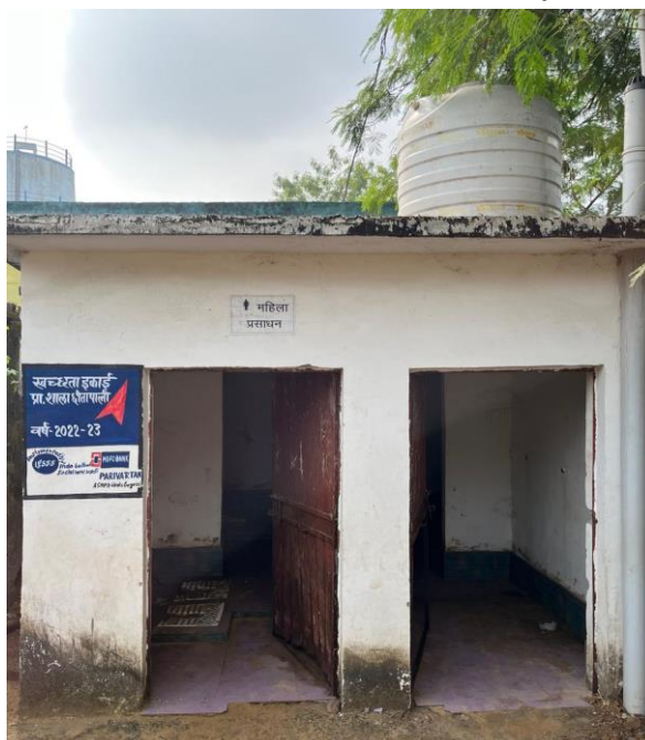
10 Toilet without water connection in Chhitapali Primary School
