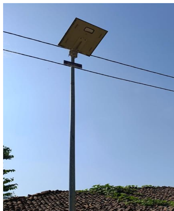
2 Non-functional Street light, Pantora
