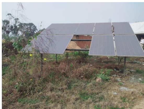
1 Non-Functional Solar Pump, Angarkhar
