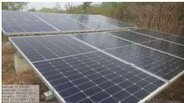
Figure 35: Solar irrigation system in Sirohi ki Bhagal
