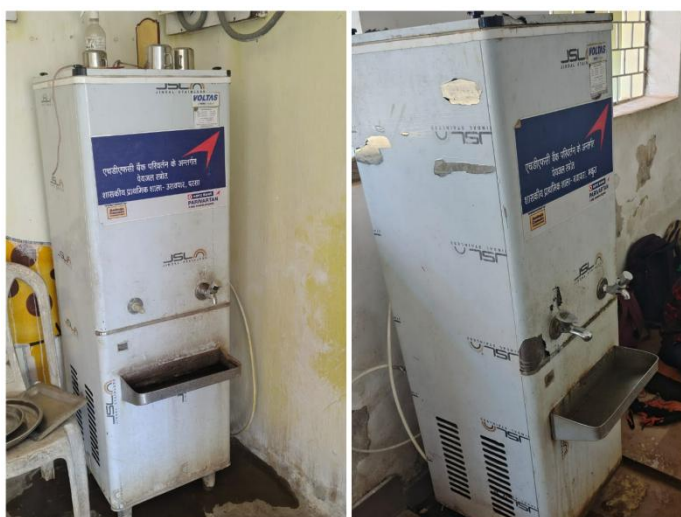
Figure 9 RO for drinking water inside school
