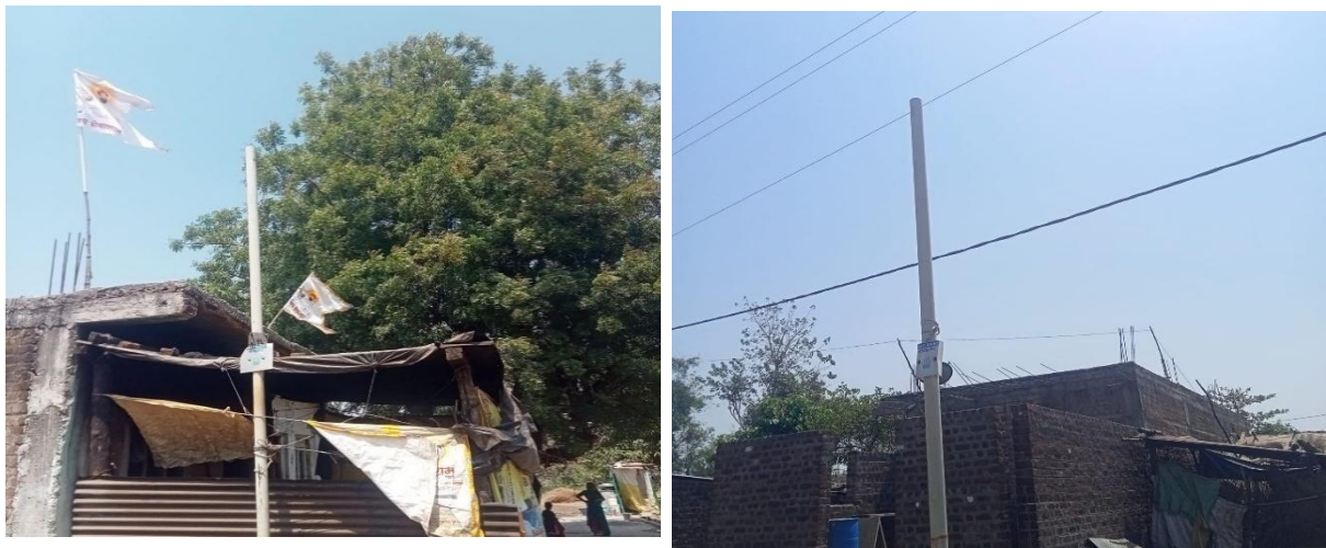
Figure 2 Non-functional Solar Street Lights
