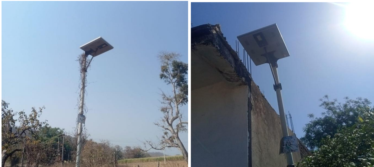
Figure 1 Functional Solar Street Lights
