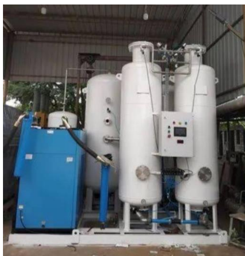
Img: Oxygen Plant, Govt. Civil Hospital Jalalabad
