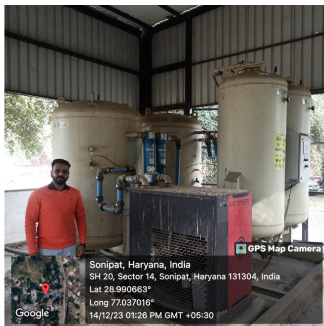
Img: Oxygen Plant, District Civil hospital Sonipat
