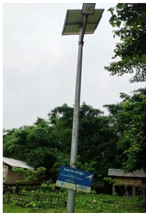
Image 7: Solar Street light setup under HRDP in Lakhimpur, Assam
