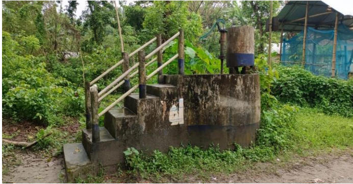
Image 6: Drinking water infrastructure built under HRDP in Bordubi Lakhimpur
