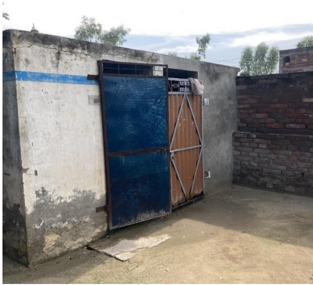
Picture 4: Toilet built under HRDP in Sodhiwala village, Punjab
