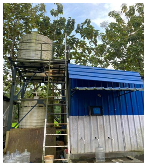
Image 3: Arsenic removal water plant
