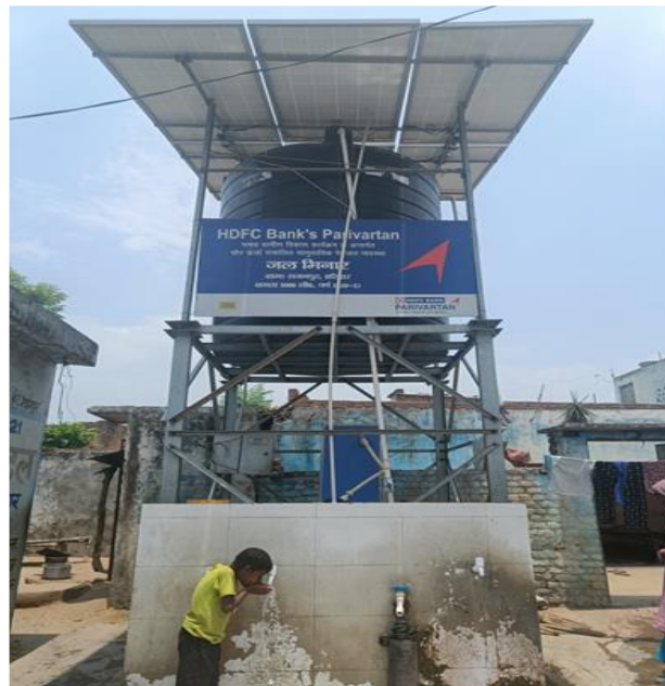
Image 5: Solar Water Tank
