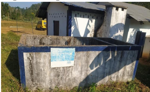
Image 12 : Garbage Bin Unit in Pahambirthem
