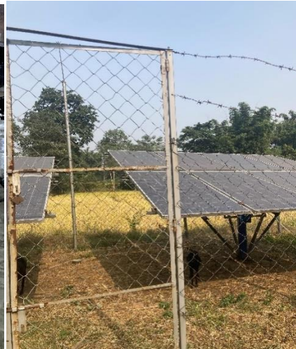
Solar Irrigation structure
