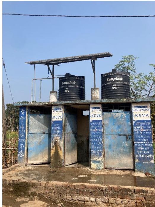
Solar Powered Bathing Units
