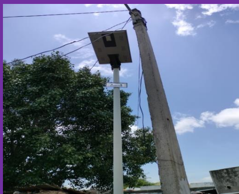
Image 7- Solar Street light installed in Pimpaldar village
