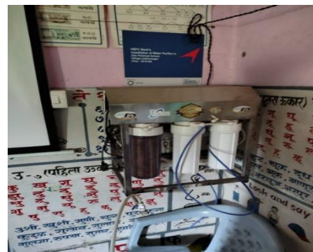
Image 11: RO unit in school, Dhawal village, Satara
