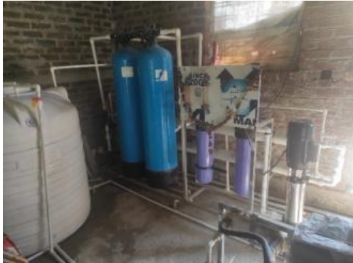
Image 9 Installation of RO filter, Varudtofa village, Washim
