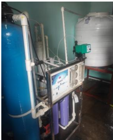
Image 11 RO filter installed in the school, Adoli village, Washim
