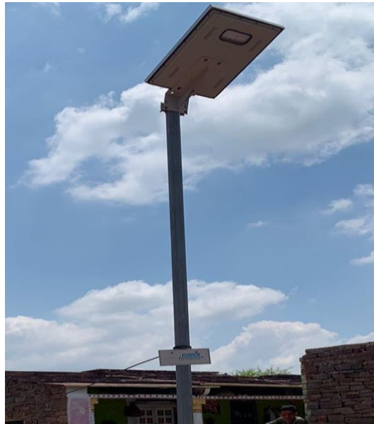
Figure 12: A Solar Light Installed in Project Village
