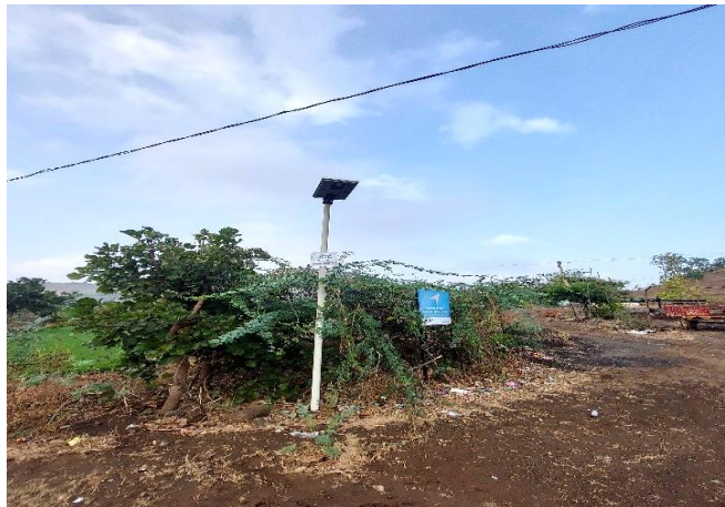
Image 4: Solar Street Light installed at Ambapani village
