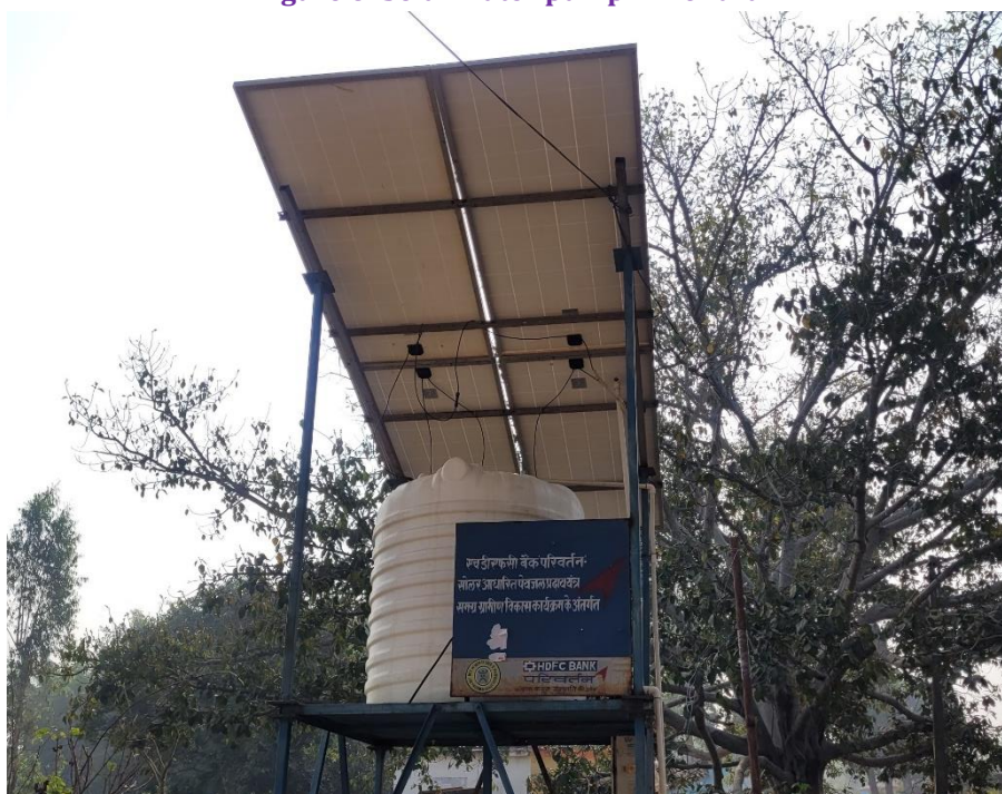
Figure 6: Solar water pump in Pendra
