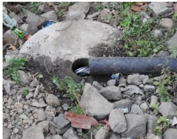
Image 4: Household wastewater soak pit
