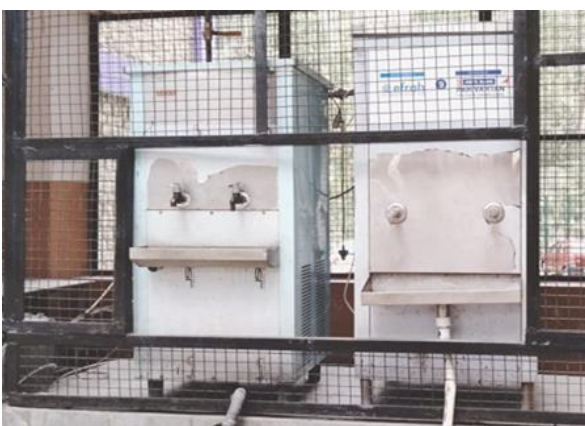
(e) Drinking water coolers
