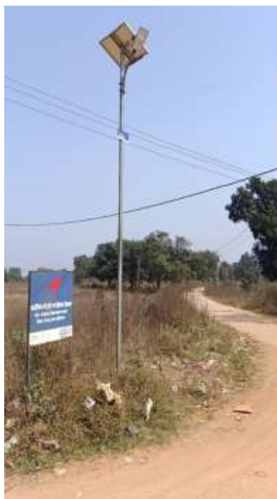
Solar light installed
