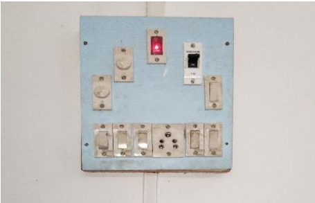
Image 2 Switchboard in smart classroom
