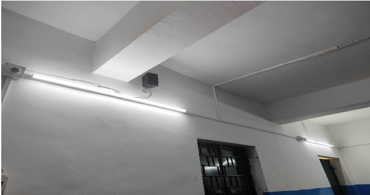
Image 3 Tube lights in Smart Classroom
